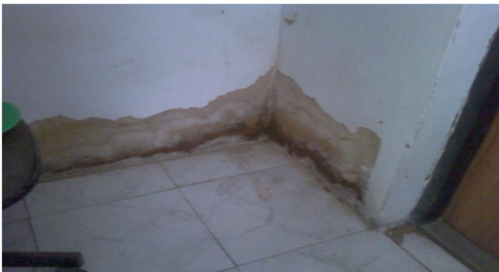
Plate 1: Damp in the sitting room
