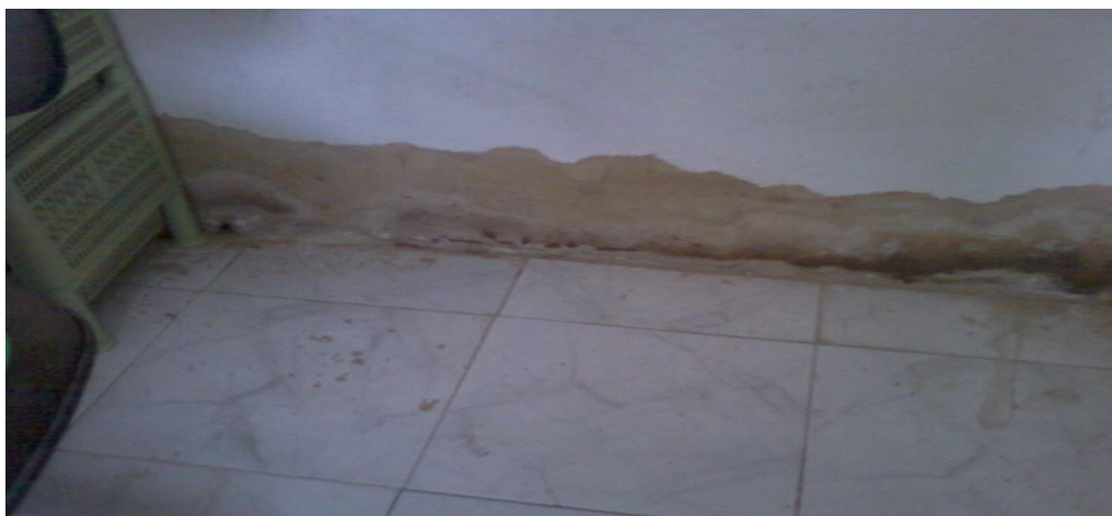
Plate 2 Damp in the kitchen
